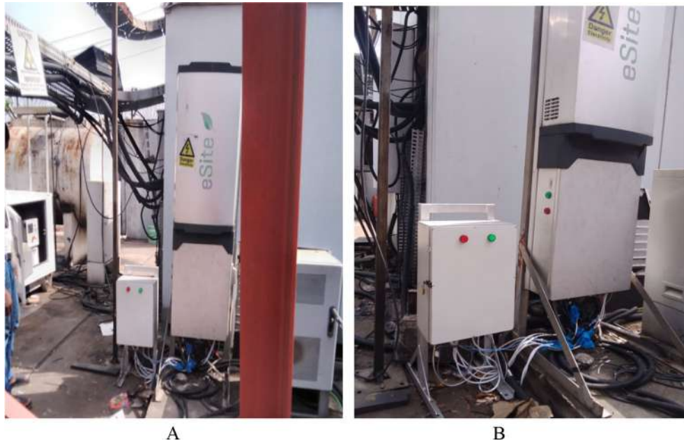
Figure 26. A: Site installation picture view 1; B: Site installation picture view 2.
